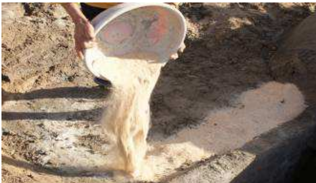
Picture 15 Using sand to give a level base for the reservoir tank
